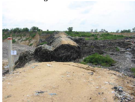
Edges of the collapse
