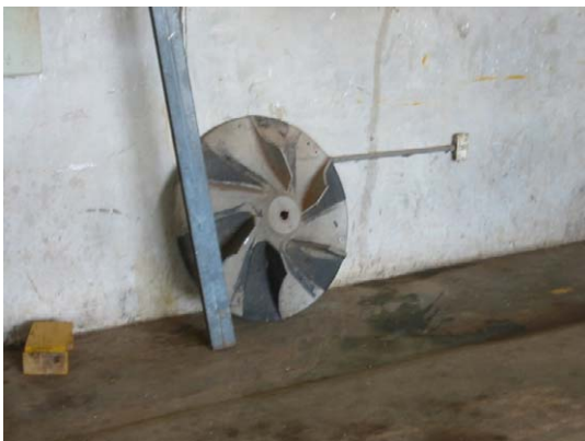
Broken part costing 3,500US$
