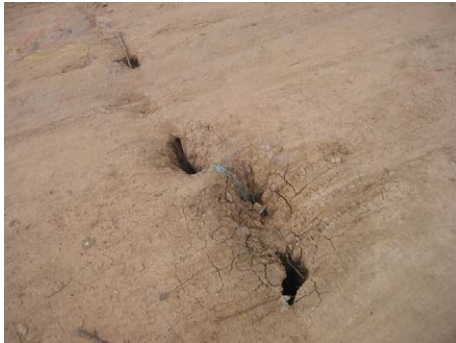
Holes Emerged on the Road Surface
