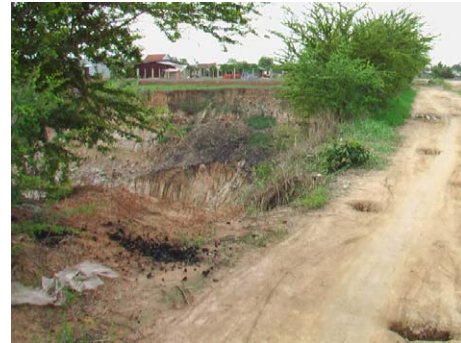
Edge of the Road Collapsed
