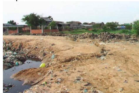
Trench on the Bank for leading water and leachate to the expansion area
