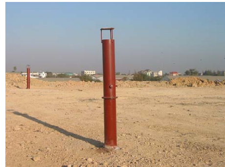
Gas Removal Facilities
