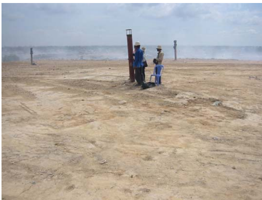
Model Block and Gas Removal Pipes
