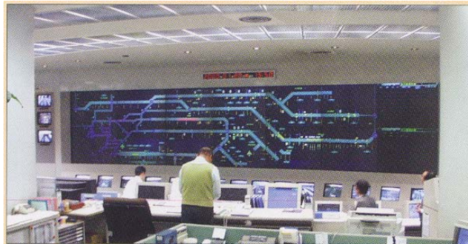
Figure 13.5-1 Example of Traffic Control Center
