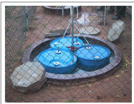
Bio-gas unit [Dutugemunu Central College]
