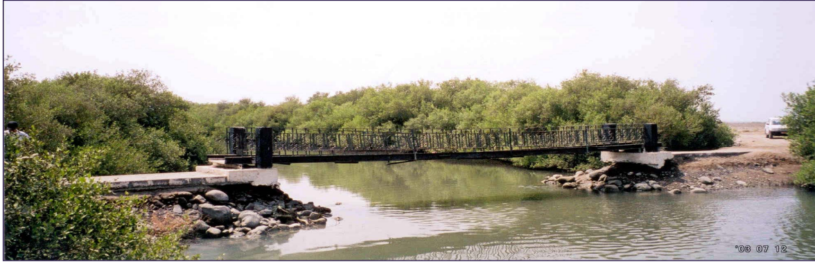
Figure 4.2.3 Khawr Shinas – environmentally damaging and unsafe construction of a bridge, illustrating need for better design of footpaths and other facilities
