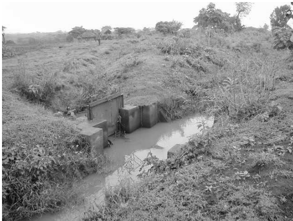
Division box with steel gate (Gidano I)
