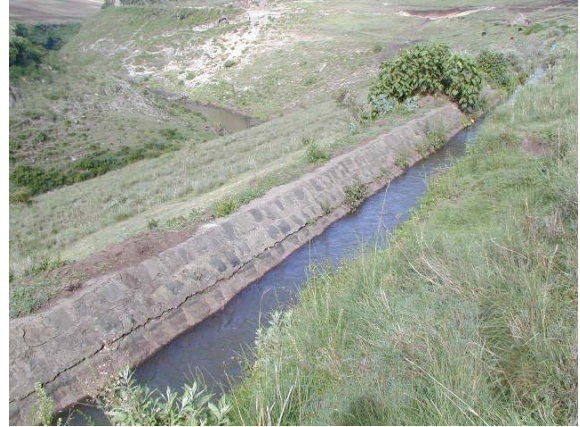
Deteriorated Main Canal with Horizontal Cracks (June 2003)
