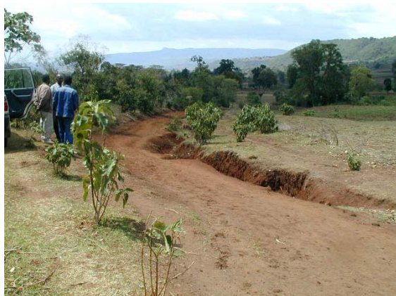
Access Road Damaged by Gully
