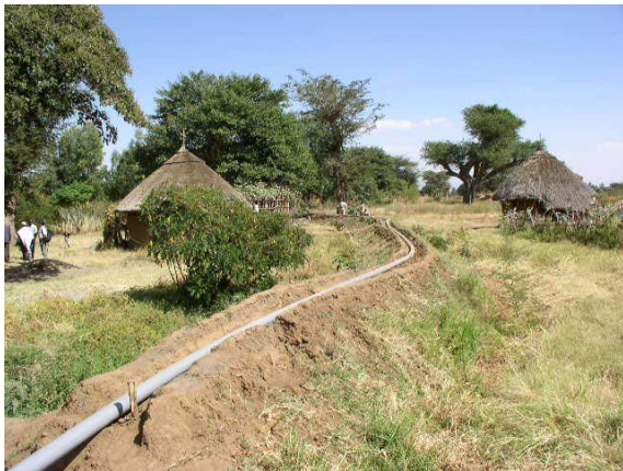
Apply of Pipeline System to Reduce Water Conveyance Loss (Oda Chisa WUA)
