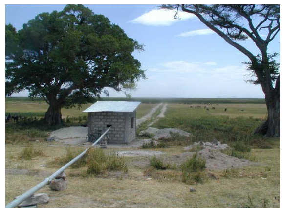
Completion of Construction Works (after 2 months from Commencement of Work, Bade Gosa WUA)
