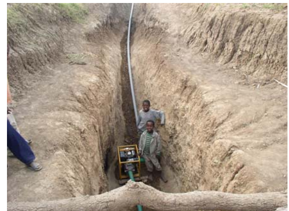
Pump Installed to Ground Irrigation Scheme (Kenteri Michel WUA)
