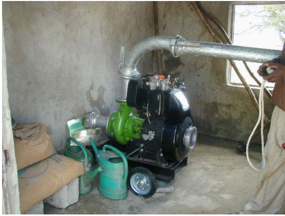
10 HP Pump installed to Schemes
