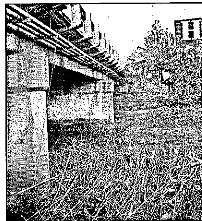
Debris at Upstream Side of Pier
