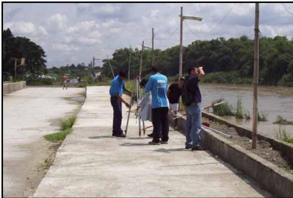
Setting up the transit that will be used for determining a right angle from the opposite bank and second observation line
