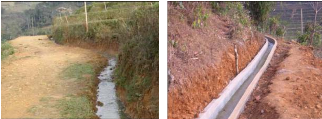
Figure 3-10 A no-lining channel (left) and a brick masonry (mortar finish) channel (right)
