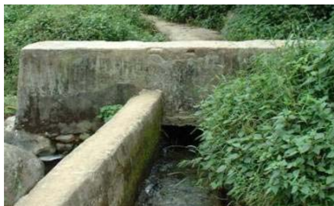
Figure 3-5 An orifice at intake to control the water flow
