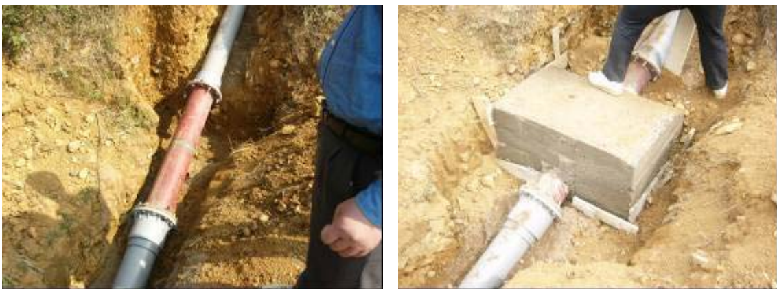
Figure 3-20 An anchor block and a steel joint pipe
