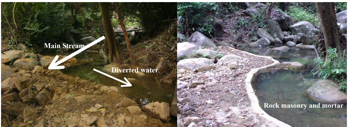
Figure 3-3 A weir and intake constructed by local technology
