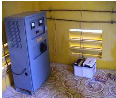
Figure 3-44 Battery charging system
