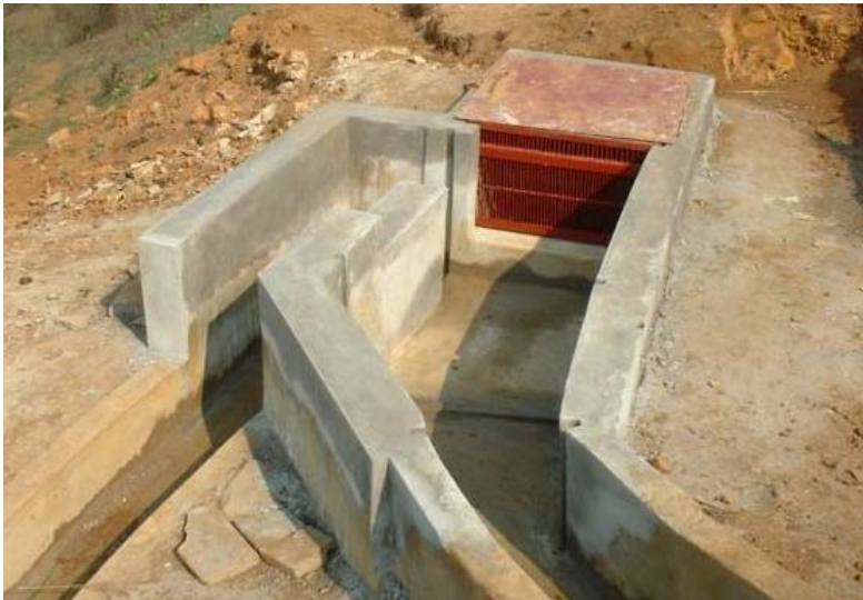
Figure 3-3-9 The head tank
