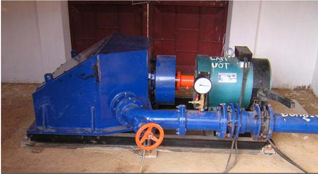
Figure 3-4-2 The turbine/generator unit: turbine casing (left) and generator(right)
