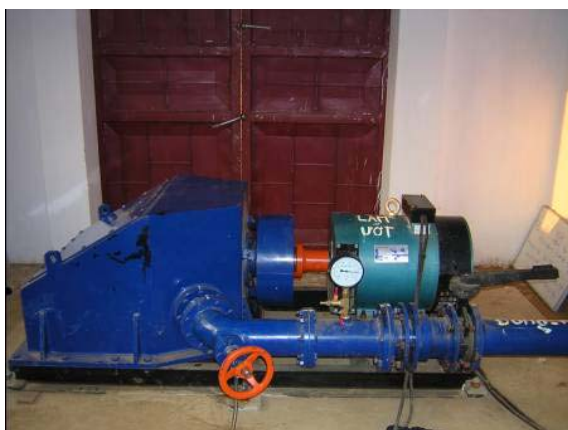
Water-turbine and generator
