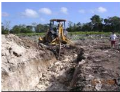
Manual Landfill Note the quality of the ground
