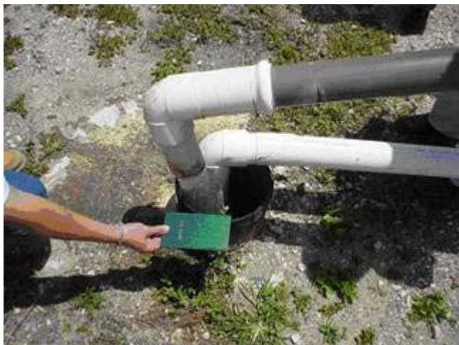
Figure C-21: Injection Well in CAPA Felipe C. Puerto
