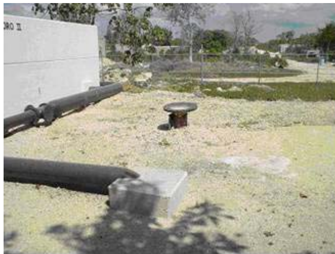
Figure C-32: Injection Well in the Treatment Plant of CAPA in Playa Del Carmen
