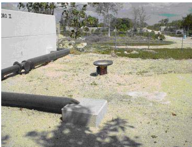
Figure 4-4: Injection Well in the Treatment Plant of CAPA in Playa Del Carmen
