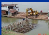
3) Putting rubble stones on mattress by backhoe on barge to submerge mattress
