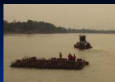
1) Towing floating Soda mattress by boat from Kao Liao stockyard into the site
