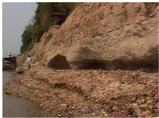
Figure 4.13 Notches Development at the foot of Riverbank Slope at Sibounheuang Site
