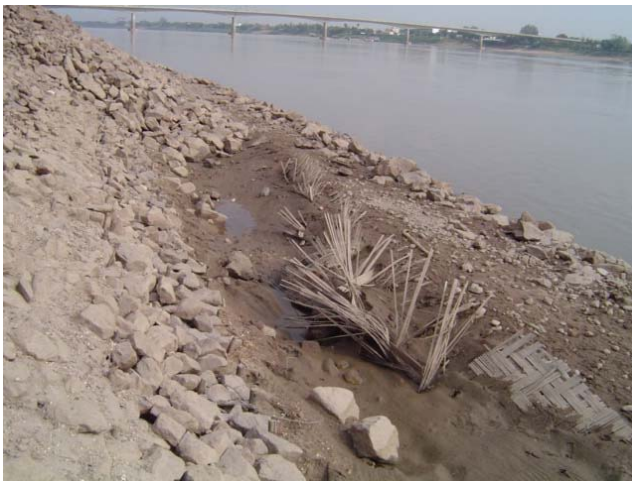
Figure 1.3 Local Scoring at the toe of Slope Protection Work
