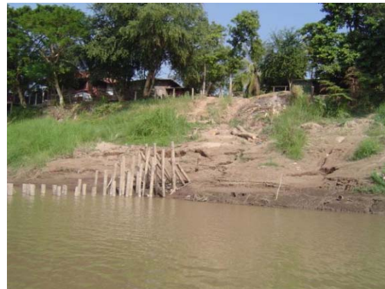
Figure 1.8 Inclination of Wooden Piles at Line No.3+40
