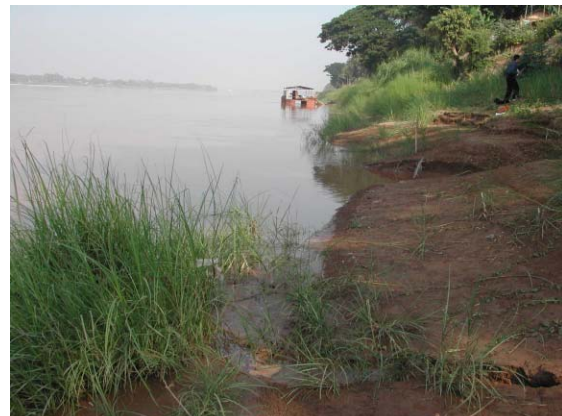
Riverbank condition in Chom Cheng site
