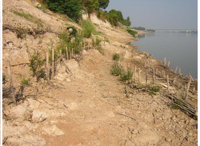
Down stream side in Nongheo site Two planting methods were conducted, Soda-net works and cutting works.
