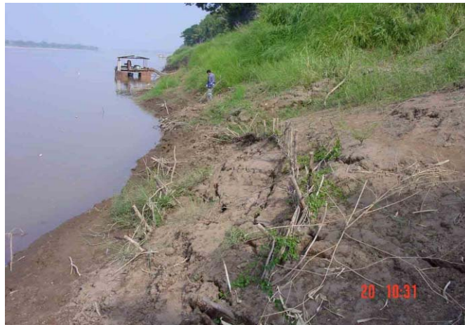
Chom Cheng site Soda-net was broken due to earth too soft.
