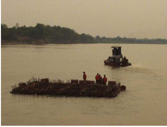
1) Towing floating Soda mattress by boat from Kao Liao stockyard into the site
