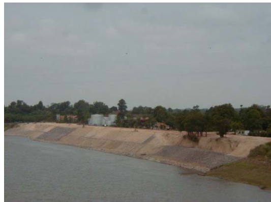
6) Overview of completed pilot works and the stone covering in front of oil tanks
