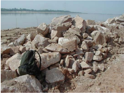
1) Crushed stone temporary stocked on the dike after transportation from the quarry site
