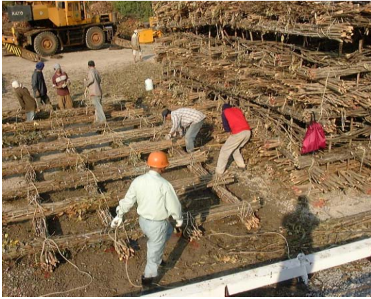
1) Arrange the tie-twig so that they form a square 1 m length fascine grid or lattice beam structure
