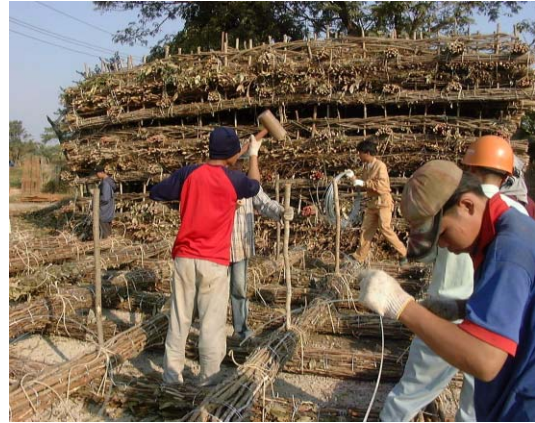
2) After assembly, the short pile will be temporarily droved at crossing points
