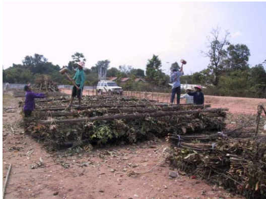
9) Piling short wooden piles to combine upper and lower lattice structures and for hurdling work
