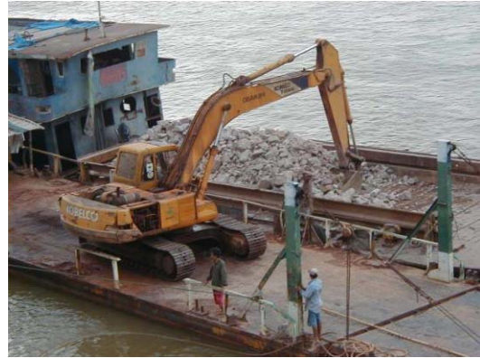
2) Stone transported from Kao Liao stockyard by barge and loaded by backhoe
