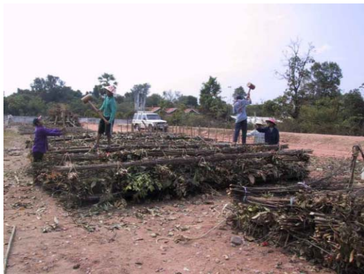
9) Piling short wooden piles to combine upper and lower lattice structures and for hurdling work
