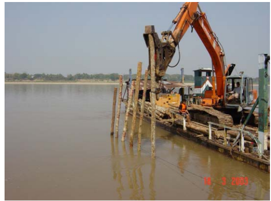
4) Piling work by backhoe with attachment to vibrate and hit a wooden log
