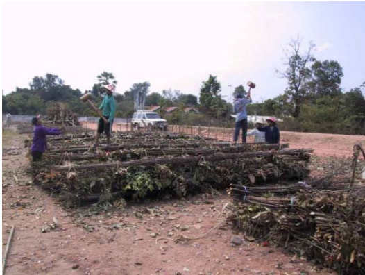
9) Piling short wooden piles to combine upper and lower lattice structures and for hurdling work
