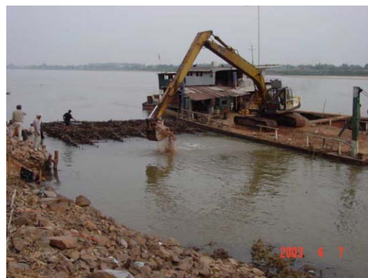
6) Putting rubble stones on mattress by backhoe on barge to submerge mattress
