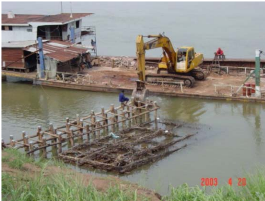
6) Putting rubble stones on mattress by backhoe on barge to submerge mattress
