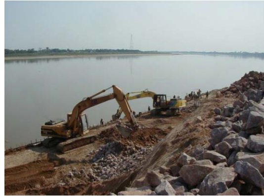
2) Stone loading by backhoe on the cat-walk level (El 161.5 m) of the lower slope
