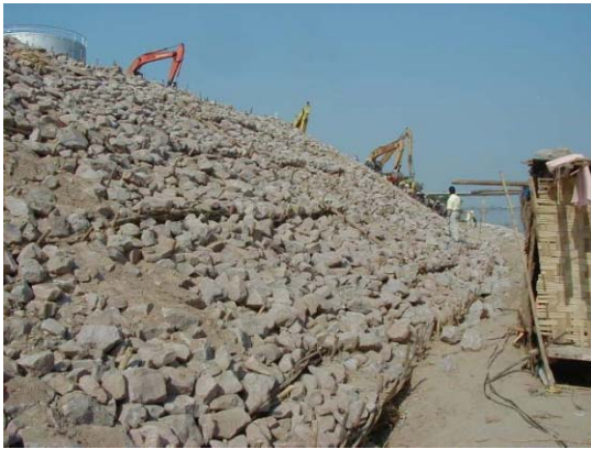
3) Stone placing by backhoe on the slope of cobble stone with willow branch work
