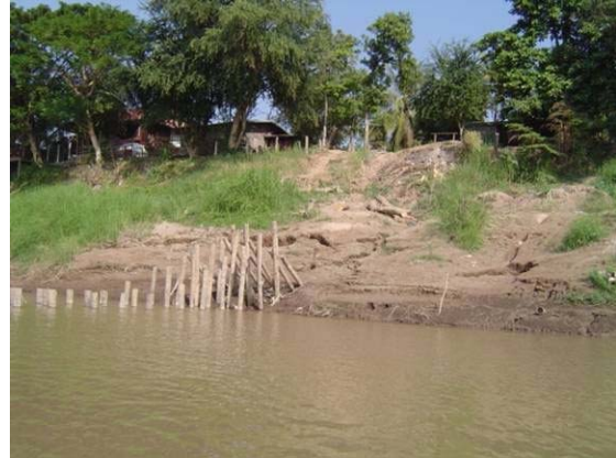
Figure 5.3 Inclination of Wooden Piles at Line No.3+40
