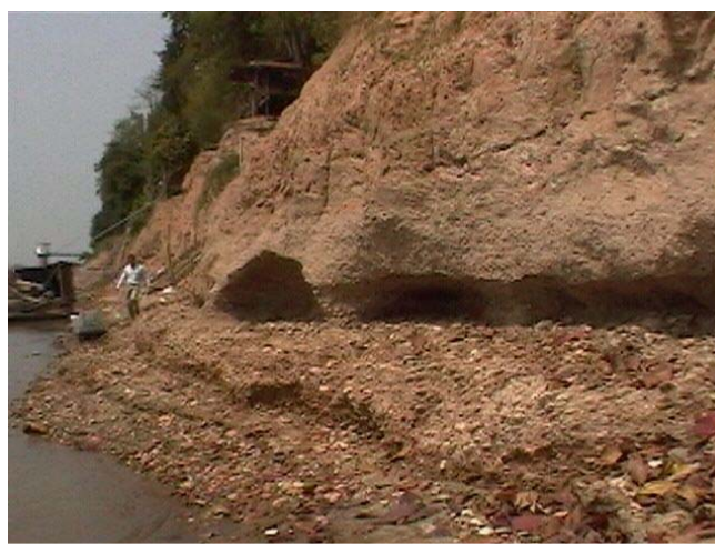
Notches Development at the foot of Riverbank Slope
