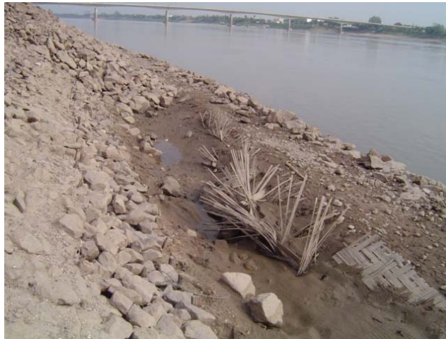
Figure 5.1 Local Scoring at the toe of Slope Protection Work
