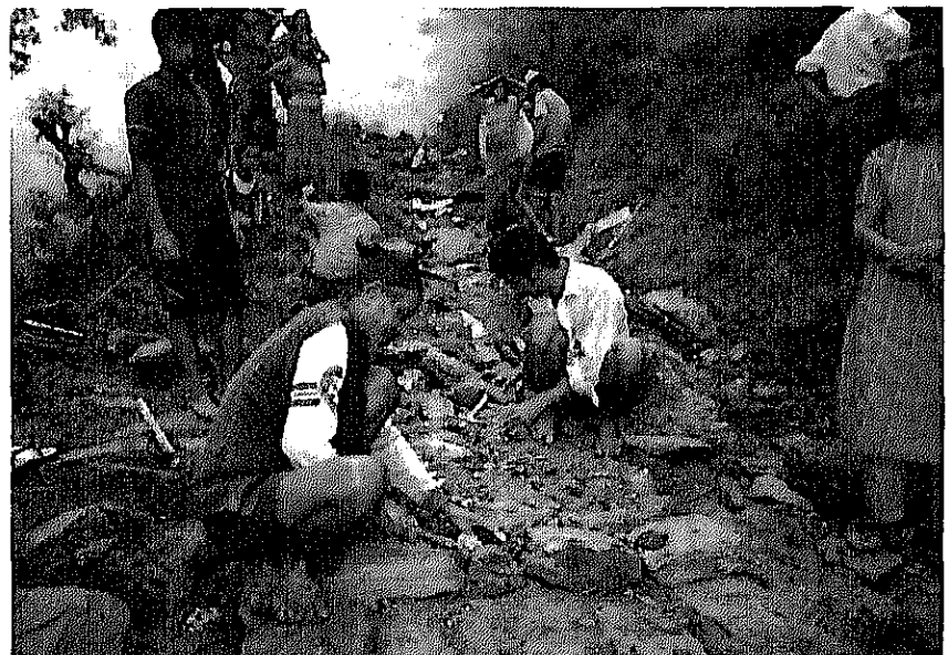
Repair work on a footpath in the Community Development and Forest/Watershed Conservation Project in Nepal
