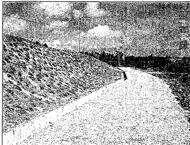
After PP (Improved slope, drainage, leachate collection (not visible) and access road)
