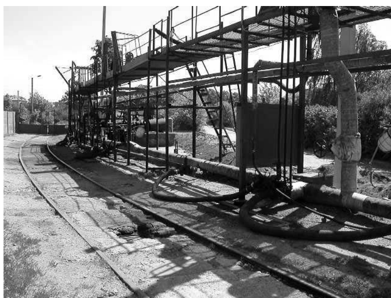
Photo I.2.5-10 Discharge Facility at Transfosa
