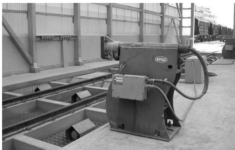
Photo I.2.5-9 Bottom Discharge Facility at Track No. 12
