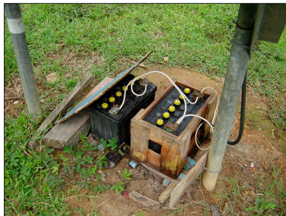
Picture B.2.2 Battery connected with BCS
