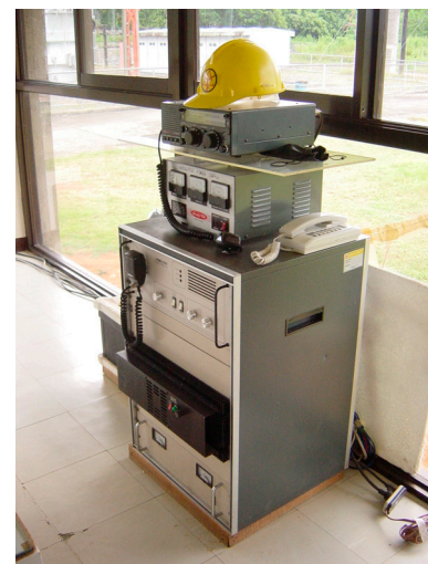
Figure 3.5.5 Radio Equipment in the Irawan Substation
