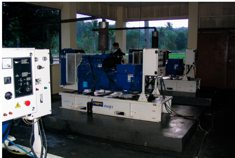
Figure 3.2.5 3 x 50 kVA Gensets
