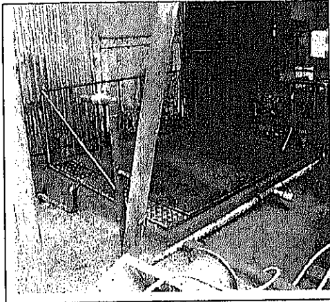
Wasted oil Storage facility
