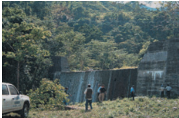
Mudslide-control dam by the “Project for Flood Control along the Choloma River”.
