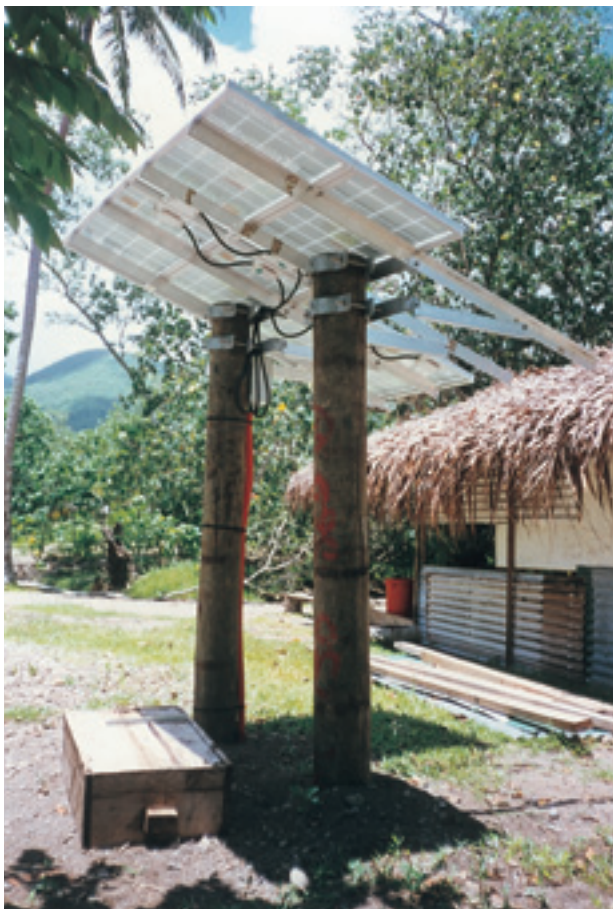
Solar Power Generation System by the “Rural Electrification Project” in Vanuatu.
