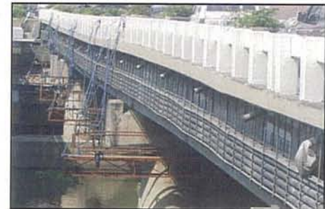
Photo 24.1.1-4 Deflection of Girders
