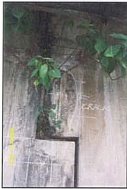
Girder 1, Gerber Hinge Damage – Crack Width 0.5mm – 1mm
