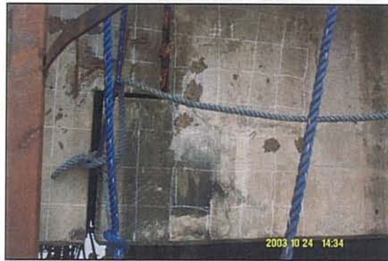
Girder 8, Gerber Hinge Damage – Crack Width 2.0mm
