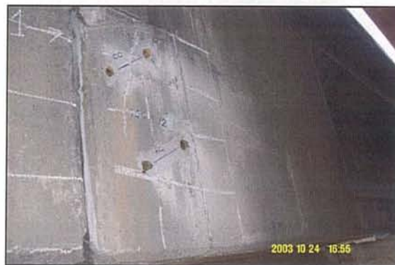
Girder 5, Gerber Hinge Damage – Crack Width 2.0mm – 5.0m
