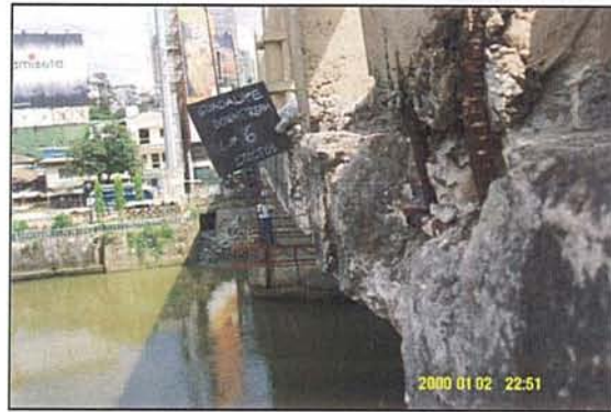
Photo 23.1.3 Sidewalk Fascia Damage – Exposed Rebar
