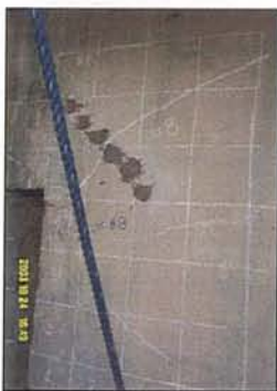
Girder 8, Gerber Hinge Damage – Crack Width 3.0mm
