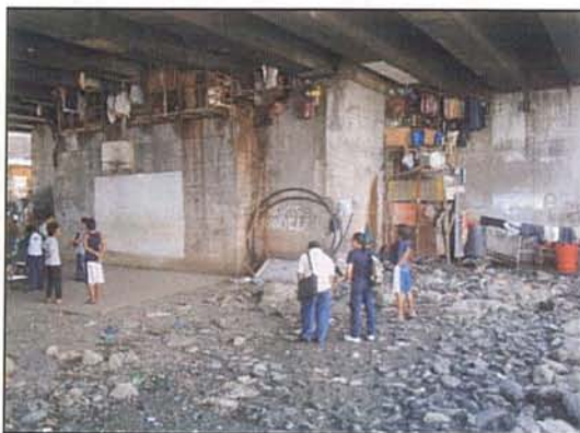
Photo 22.5.3-1 Photos showing the informal settlers' dwellings below the Lambingan Bridge columns and between the girders
