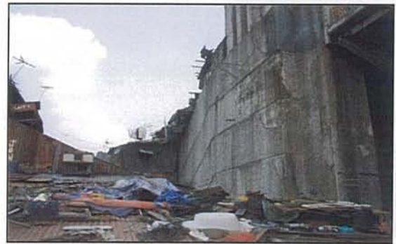
Photo 21.5.3-4 Here is where the makeshift dwellers keep their materials during day time (side of bridge)
