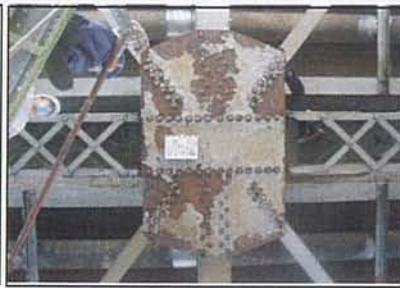
Photo 21.1.3-11 Gusset Plates, Damage – Corrosion 10 □ Section Loss < 30%
