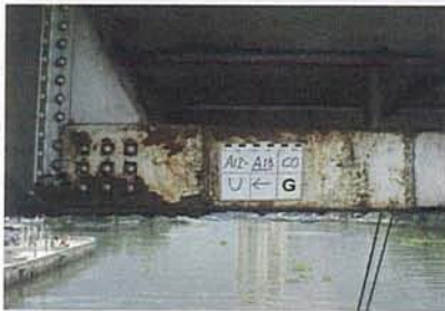
Photo 21.1.3-13 Longitudinal Tie Beam, Damage – Corrosion 10 □ Section Loss < 30%
