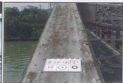
Photo 21.1.3-15 Arch Top Chord Damage – Corrosion Section Loss < 30%
