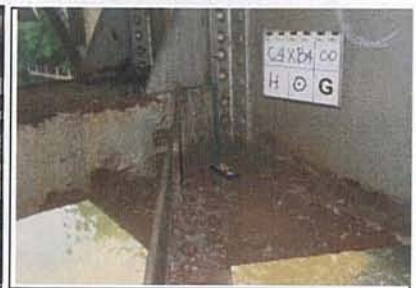
Photo 21.1.3-12 Deck Frame End Braces, Damage – Corrosion Section Loss □ 30%
