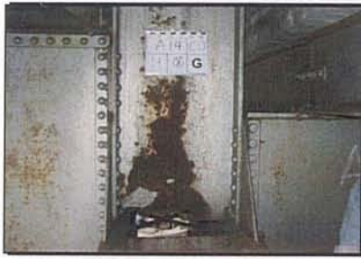
Photo 21.1.3-10 Vertical Hanger, Damage-Corrosion 10 □ Section Loss < 30%
