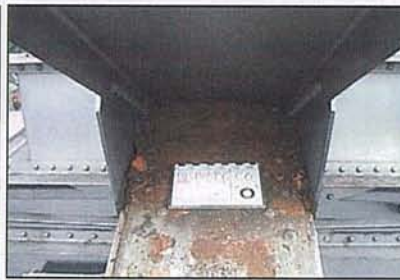
Photo 21.1.3-14 Arch Bottom Chord, Damage – Corrosion 10 □ Section Loss < 30%
