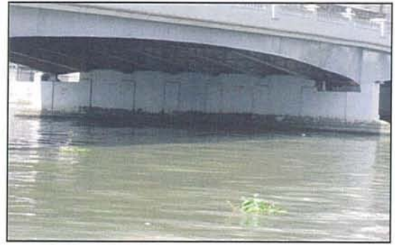
Photo 20.1.1-2 Shear keys as shown on Top of Piers and Abutment are part of ERP Retrofit Program in 1997.
