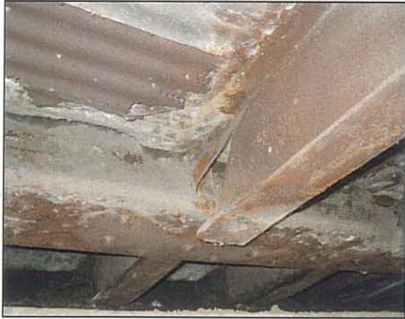
(a) Fractured Stringer and Heavily Corroded Cross Beams
