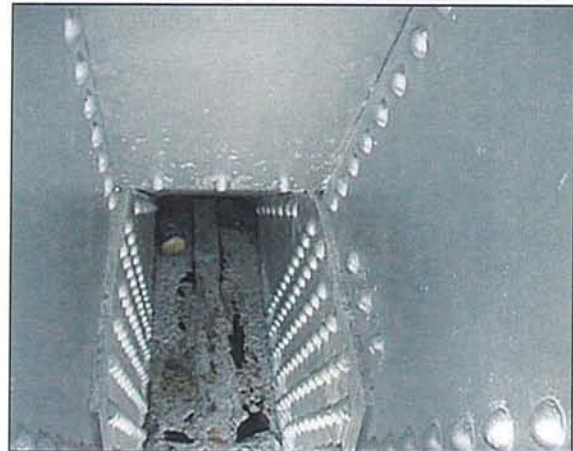
(b) Reduced cross section of Bottom Chord due to corrosion
