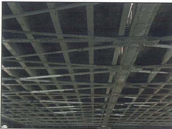
Photo 13.3.1-3 Below Deck Level - Bottom Chords, Cross Beams, Stringers, Deck Bracing and Gusset Plates. North Span shown (Looking South)
