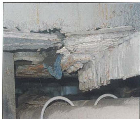
(d) Heavily Corroded Stringer at South East
