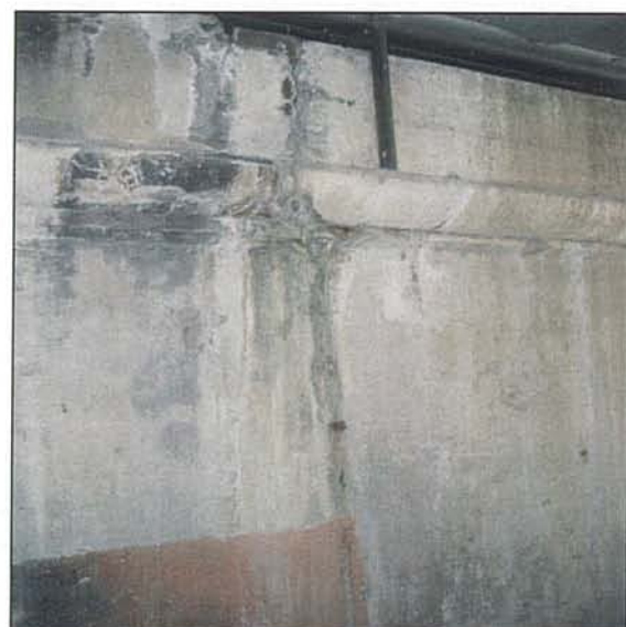
(f) Cracks and Concrete Spalling at Abutment (View South)
