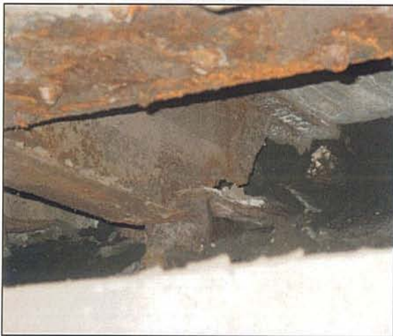
(c) Fractured Stringer at North East Portion
