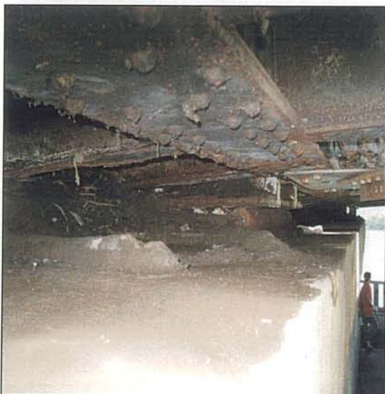
(e) Damaged at Substructures and Bearings, Corrosion and (Abnormal) movement of Bearing at North Abutment. Roller most likely stuck-up
