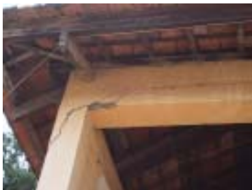
Cracked Pillars and Beams of One-Story Classroom Building
