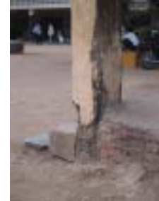
One-Story Classroom Building with Reinforcing Bars Exposed
