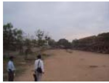
Construction Site for Project Classroom Building Site control is required in that the site is sloped with slight grade
