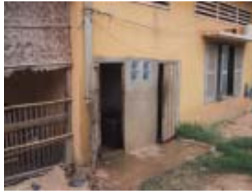
Toilet Facilities for Pupils Newly built at the space underneath staircases after the Basic Design Study
