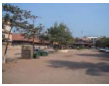
Construction Site for Project Classroom Building Upper parts of the decrepit buildings to be demolished have been removed. The foundation still remains.
