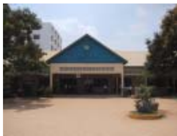
Existing Administration Building Planned to be demolished in the Basic Design Study, but will continued to be used with thorough repair
