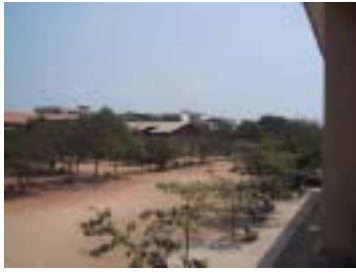
Construction Site for Project Classroom Building Upper parts of the decrepit buildings to be demolished have been removed. The foundation part still remains.
