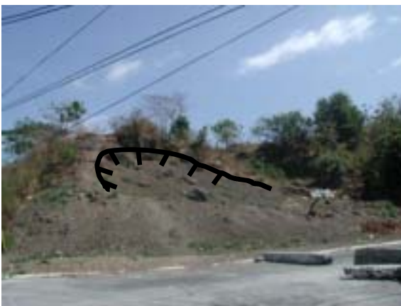
Picture-5 Surface Failure
