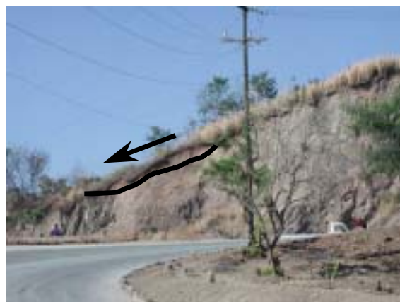
Picture-6 Surface Failure, Distribution of Weathered Zone
