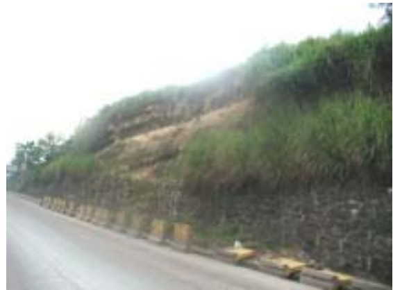
Picture-4 No Slope Protection Work
