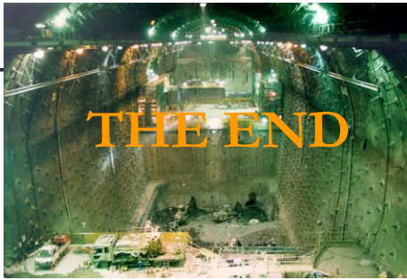
Underground Power House Cavern
