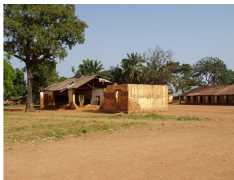
Example of Irreparable Classroom Building (3) The building is not currently used. As the walls and roof have mostly collapsed, repair work cannot guarantee structural safety.
