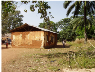
Example of Repairable Classroom Building (2) Despite general deterioration, the sound structure means that this building can be repaired.
