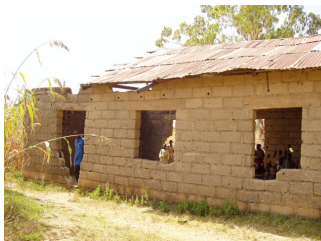
Example of Irreparable Classroom Building (2) Even though the building is currently in use, parts of the walls have collapsed. Repair work cannot guarantee structural safety.
