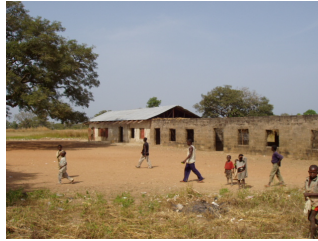
Example of Repairable Classroom Building (1) The roof of half of the building (left-hand side) has been restored by the local community. The right-hand side of the building still lacks a roof but can be repaired.
