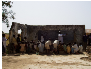
Example of Irreparable Classroom Building (1) Even though this building is currently in use, the roof and the walls have collapsed. Repair work cannot guarantee structural safety.
