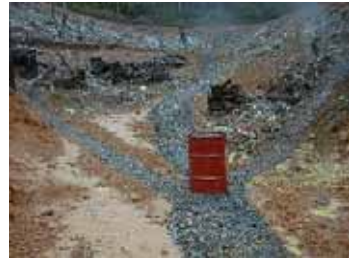
Gas ventilating facility
