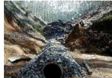
Leachate collection facility
