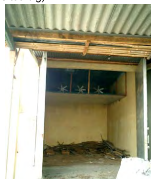
(Inside, difficult to keep hot air)
