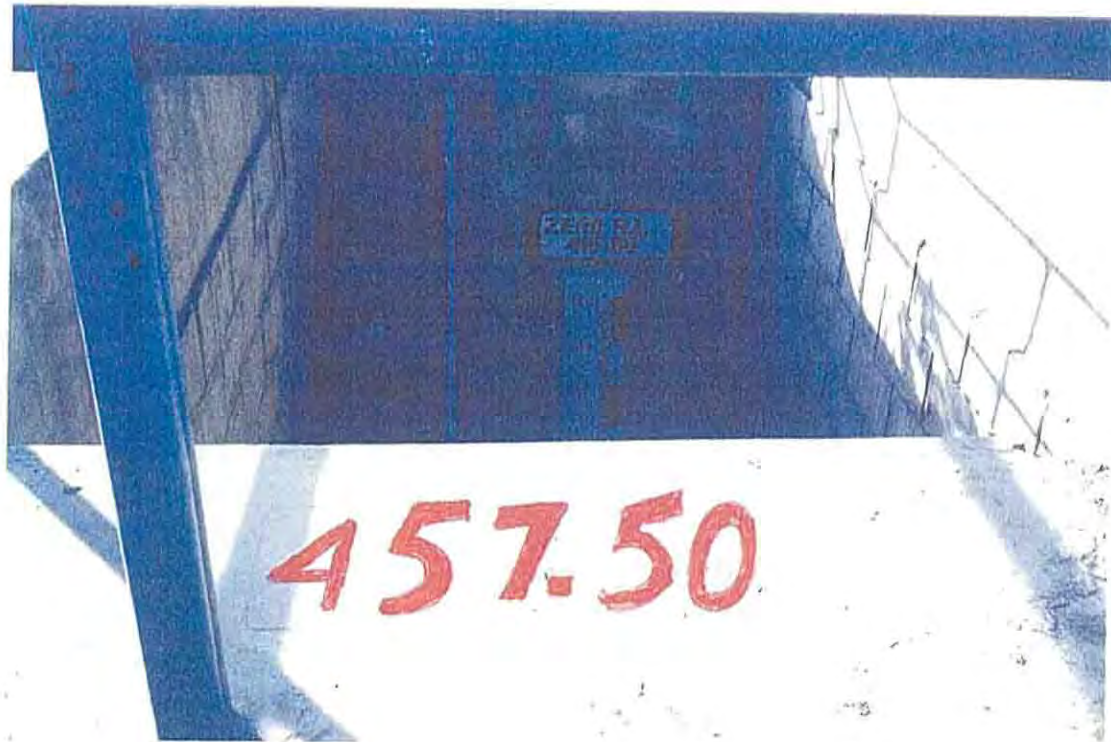
Benchmark established by the Executive Engineer Taunsa Barrage on the northern of gauge well structure Situated at D/S, of left abutment of Taunsa Barrage.
