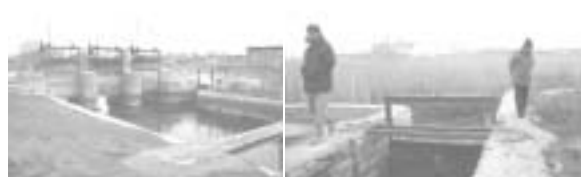
Diversion Weir ( from upstream side) Left Canal Intake (from downstream side) This weir locates in Ravansar City, just 1.0km down from the Ravansar Spring. " irrigation canals extend to both right and left sides for each I&D schemes.
