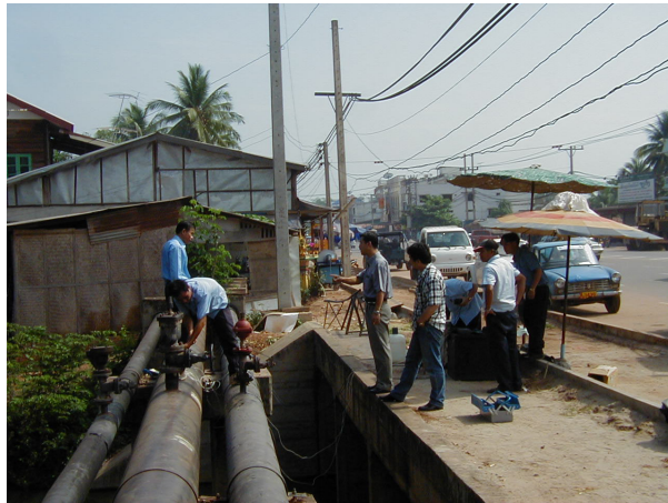
Photo A10-1 Flow Measurement at No.3, 02/04/03
