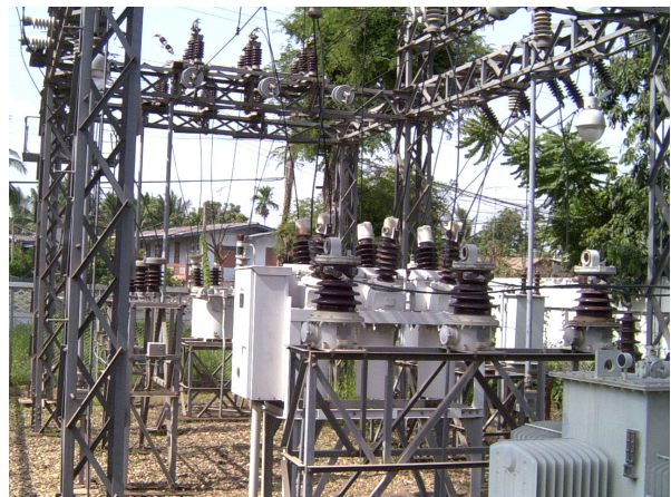
Power Sub-Station Constructed in 1964
