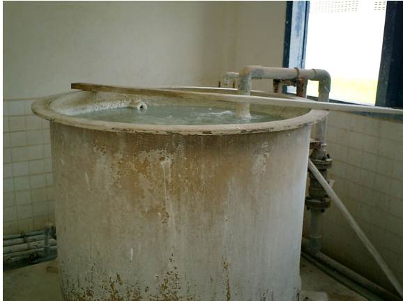
Deteriorated Hypo Solution Tank
