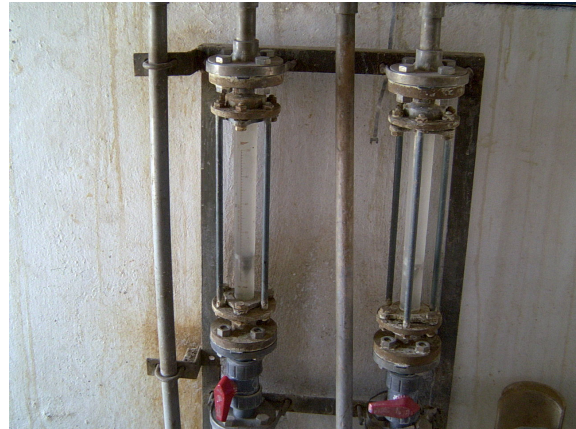
Deteriorated Alum Flow Meter
